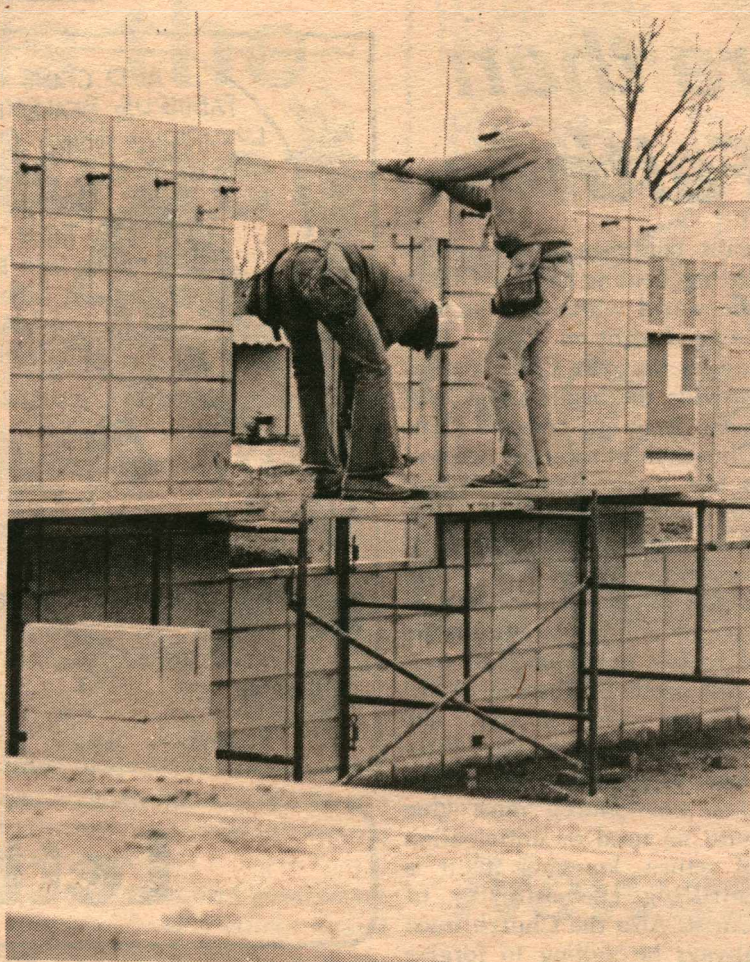
Benefiting from the great weather recently, construction of the new housing complex is back on schedule and should be ready for fall students.
