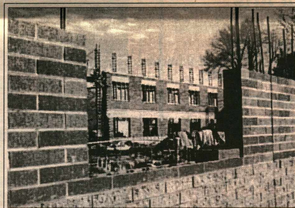
View of new freshman dorm from soccer field; construction began during first term (Diehl).
