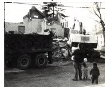
Pastor Jonathan Hoagland, Archbold, Ohio, looks on with some children as their church is demolished in preparation for a new building.
